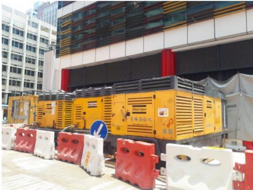
Figure A: Air compressors at Zone D3
