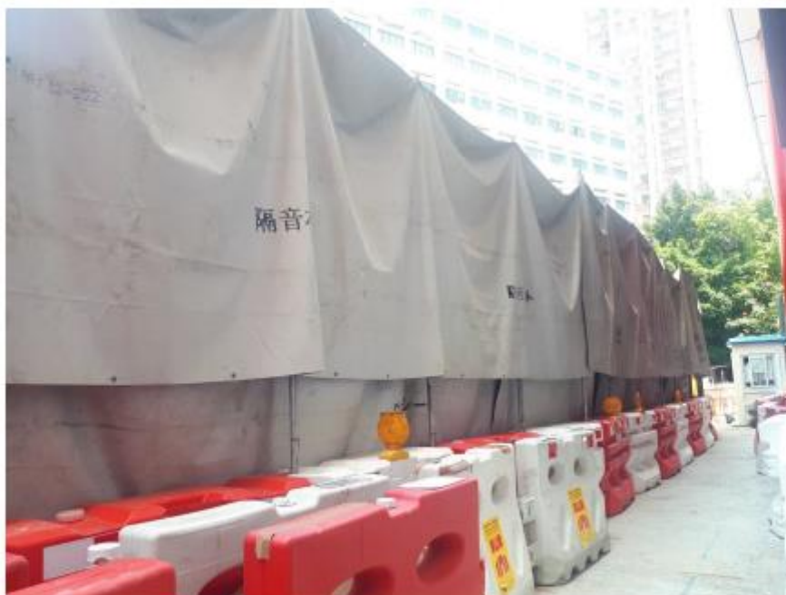
Figure B: The height of two layers of noise barrier mat near the air compressors had been extended
